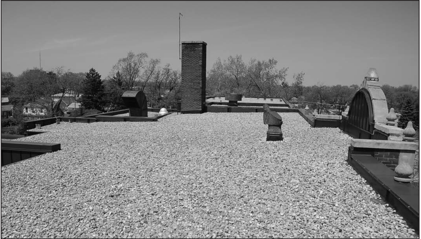
Photo 1 – Roof designers in the past strived to keep all equipment and foot traffic off of the roof. This 22-year-old ballasted EPDM roof is in excellent condition, in part because of the lack of rooftop activity.
